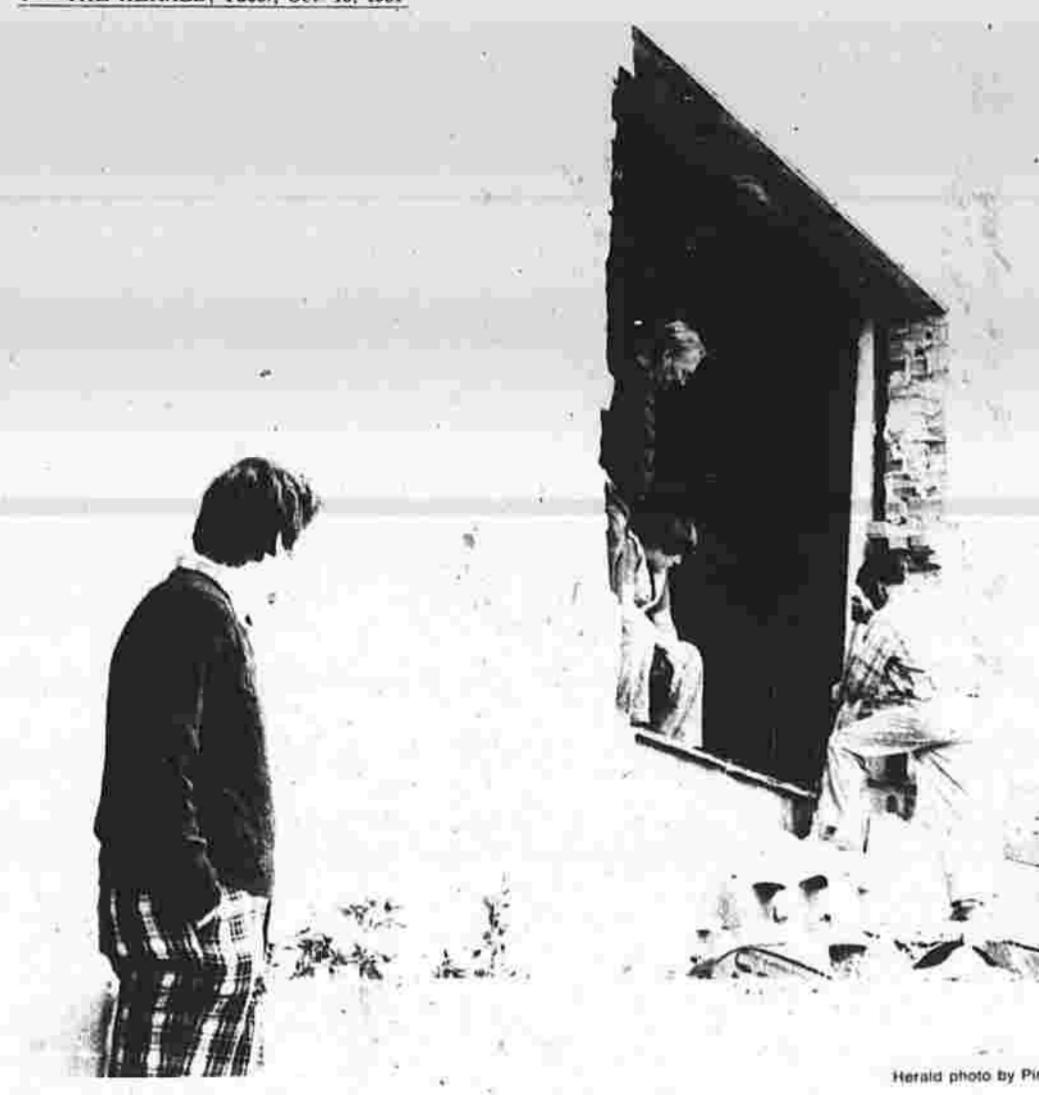
Hole in the mall Kenneth Burkamp, left, owner of the Manchester Mall at 811 Main St., watches as men work on a hole in the wall of the mall as part of the exterior renovations for a restaurant which will occupy the ground floor of the former W.T. Grant building. The workmen are (from left) Gene and John Arsenault and Norman Nicotera.
